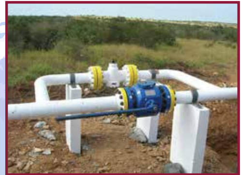
6" 600 ASME with 6" Bypass Line Tamaulipas, Mexico
