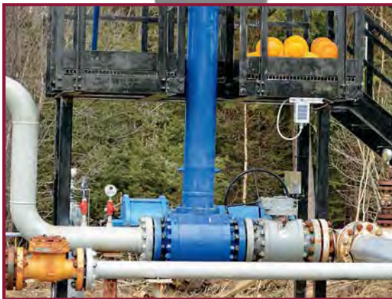
Alberta, Canada 8 inch 600 ANSI, seven pig capacity Pneumatically actuated
