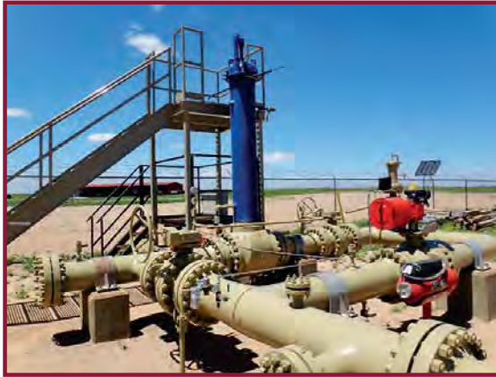
Colorado, USA 12 inch 600 ANSI, five pig capacity Pneumatically actuated
