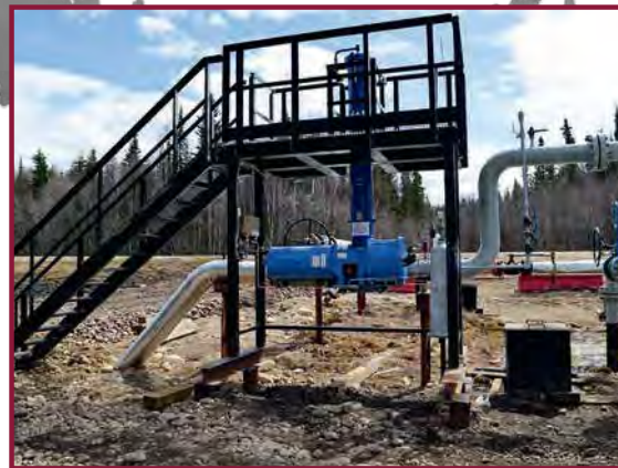
Alberta, Canada 6 inch 600 ANSI, seven pig capacity Pneumatically actuated
