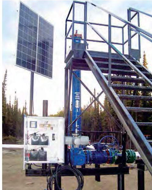
Alberta Canada, 6" 600 ANSI, eleven pig capacity, self-contained solar electric actuation
